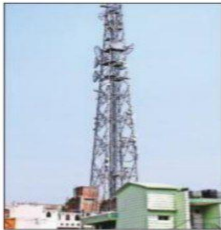
BSNL towers, Jammu. File
