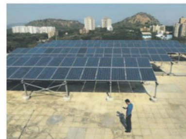
The panels will be set up in CAPF, NSG campuses.
