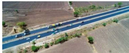
In one shot: Part of the 75-km bituminous single-lane road laid in 105 hours, 33 minutes. ■ANI
