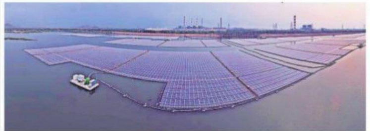
The floating solar plant at Ramagundam: 500 acres, capacity 100MW. NTPC
